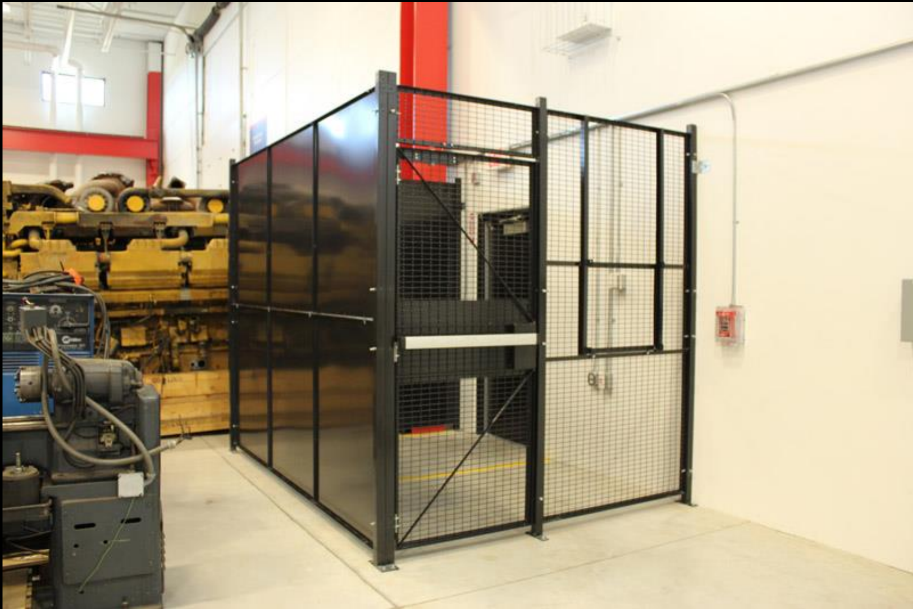
Driver & Building Access Cages
